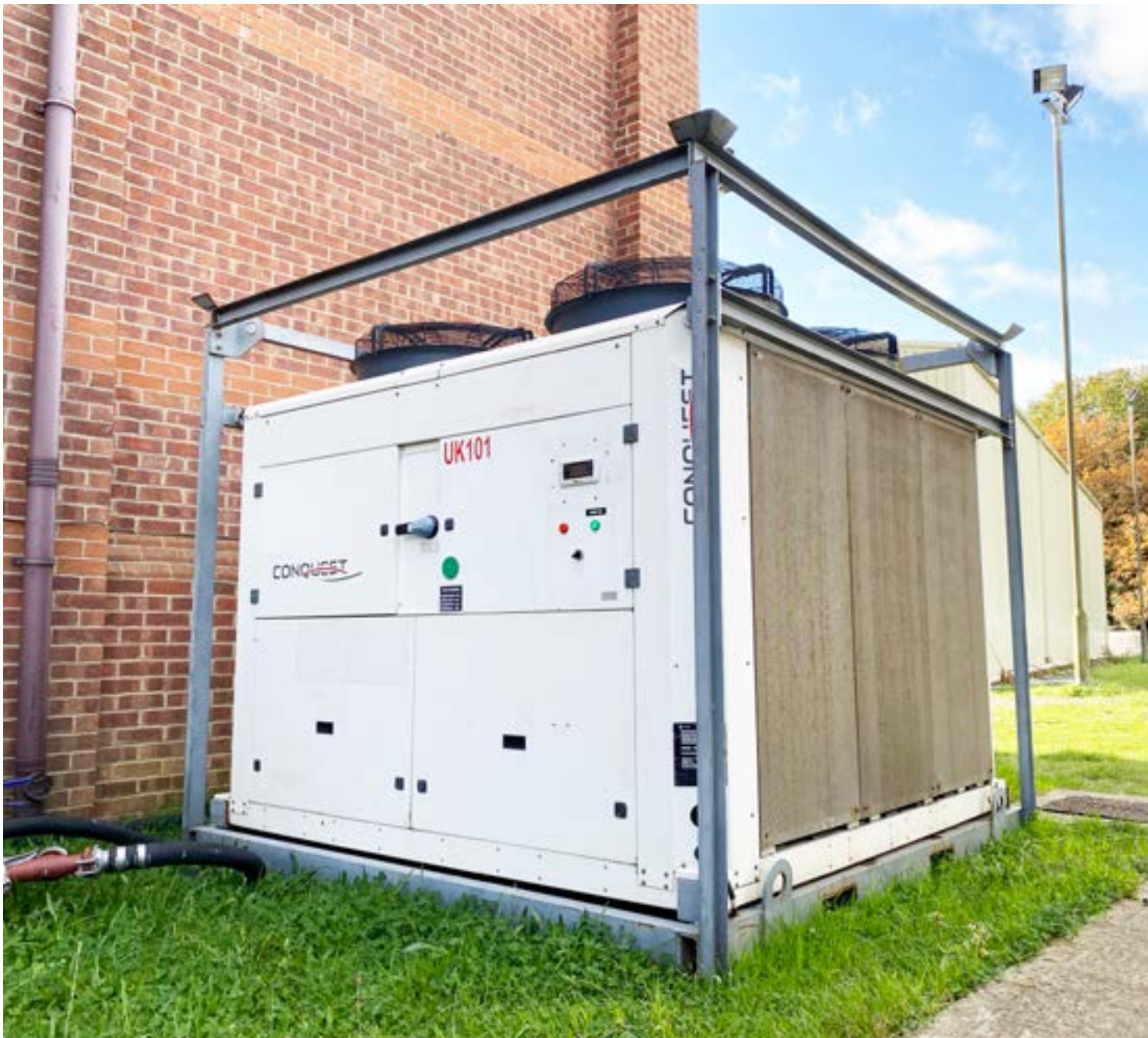
HVAC systems for stages and workshops
